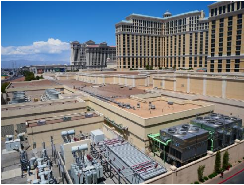
Bellagio Hybrid Cooling Tower
